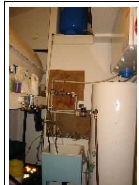
Fig. 22: cistern, HWT, HRV
